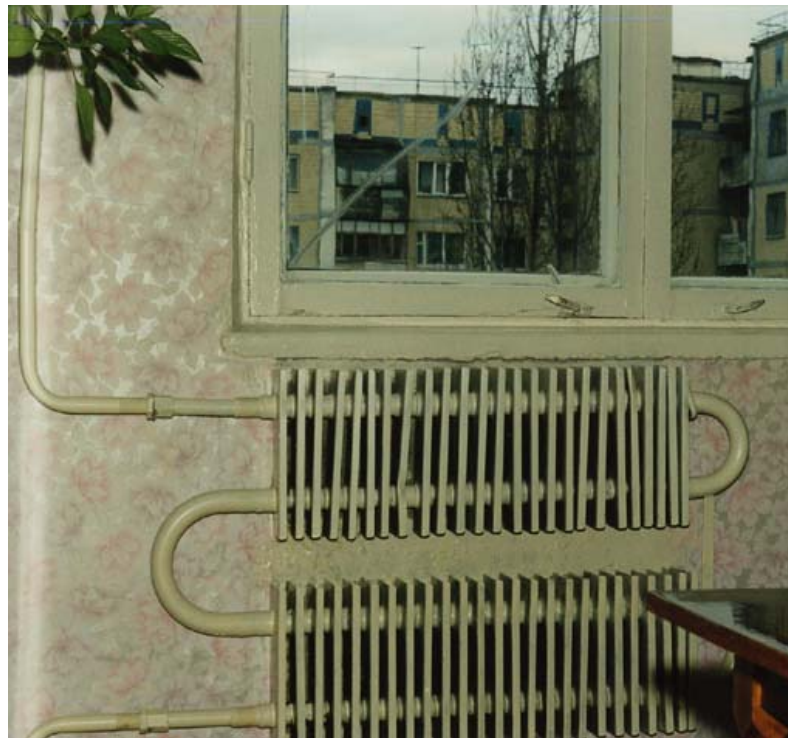
Battery of Heating
