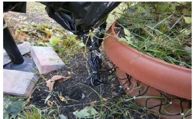
Buried Coaxial Cable and Buried Counterpoises
