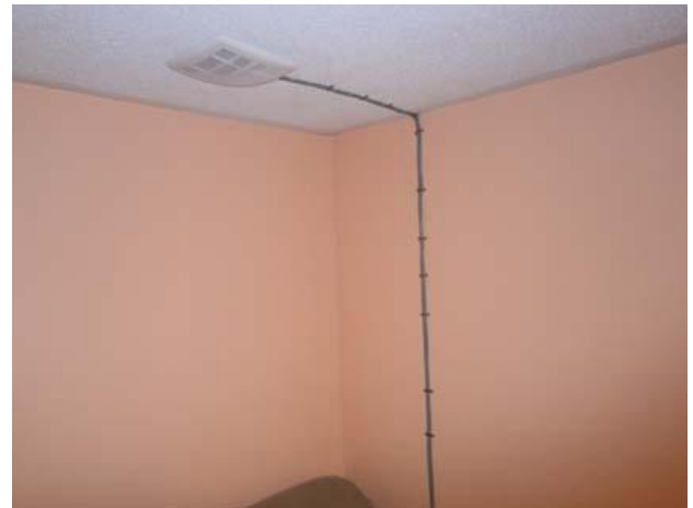
Picture 5 Coaxial Cable going into my Basement
