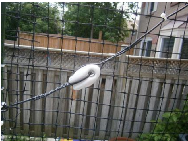
Photo 7 Insulator at the end of a slope wire
