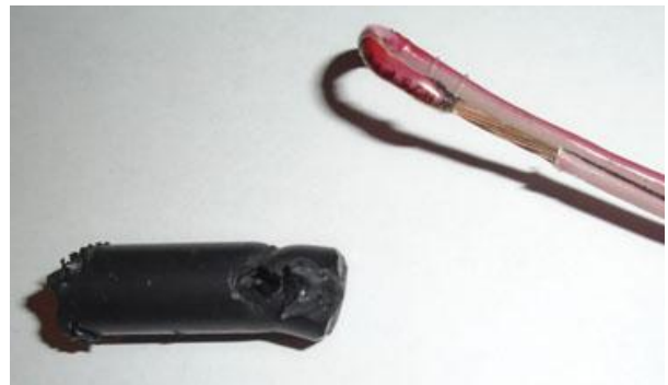
Molten Insulator and Guy with Melted Insulation
