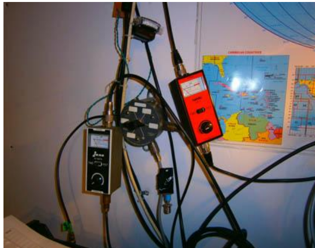
Photo 6 SWR Meter at the Antenna Cable
