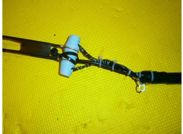
Photo 4 Coaxial Cable Connection to the Two Wire Line
